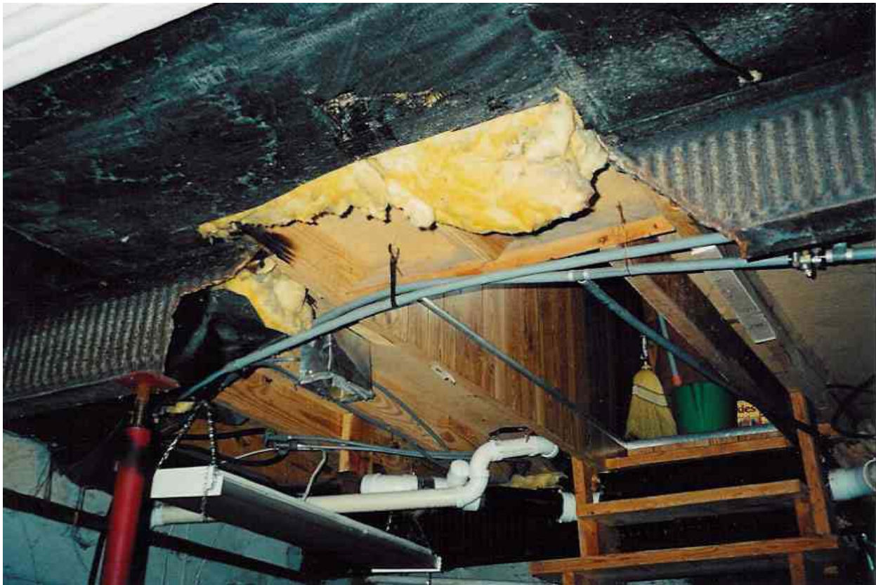
(c) Area of trailer floor beam with portion removed from stairway
