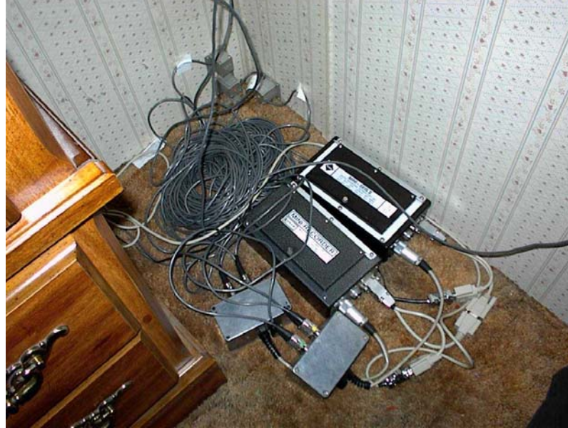
Figure 2.2 Typical S1 cluster of transducers in the lower corner with S1 and S2 seismographs
