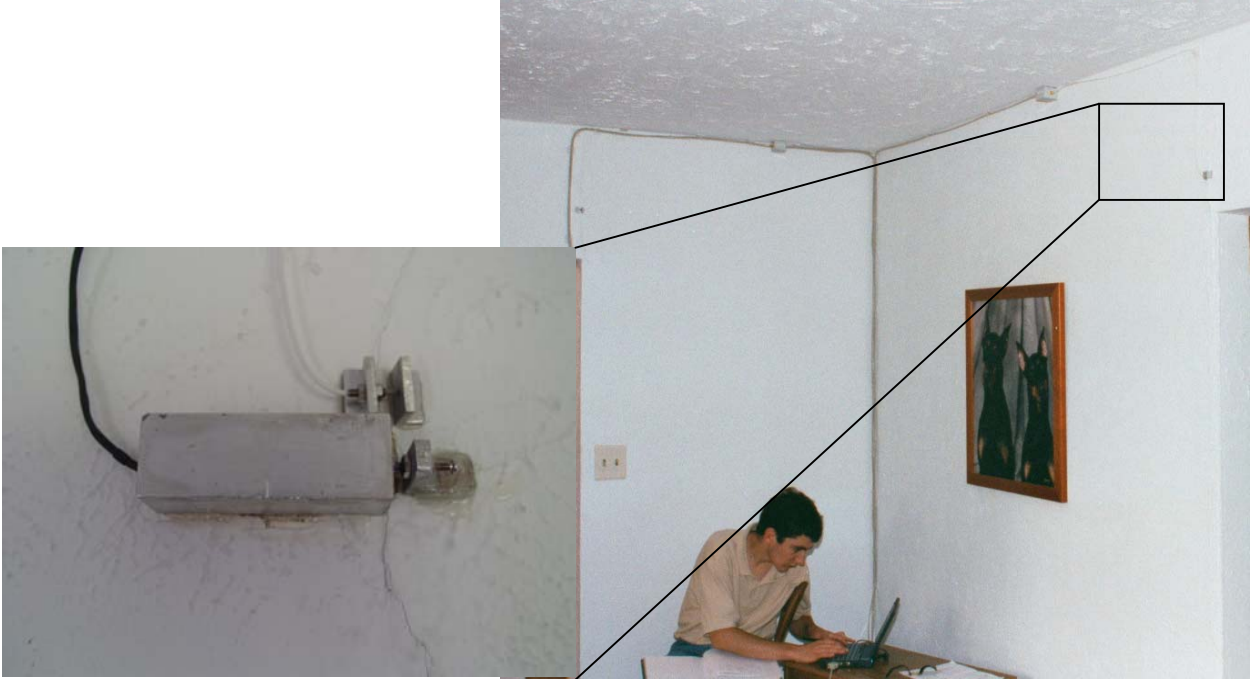
Figure 7.3 Kaman and LVDT displacement sensors spanning Crack 1
